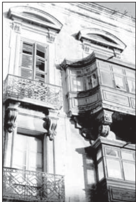
Derelict building at the corner of Merchants Street and St Lucija Street
