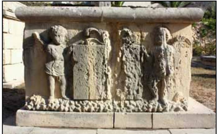
Stonework requiring restoration at Msida Bastion Cemetery
