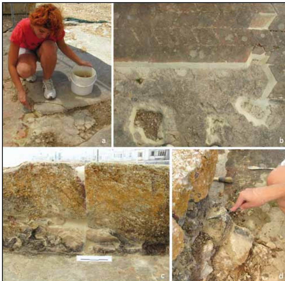
A sequence of photographs taken during the emergency conservation treatment carried out at the Żejtun Roman Villa in August and sponsored by the HSBC Malta Foundation.
