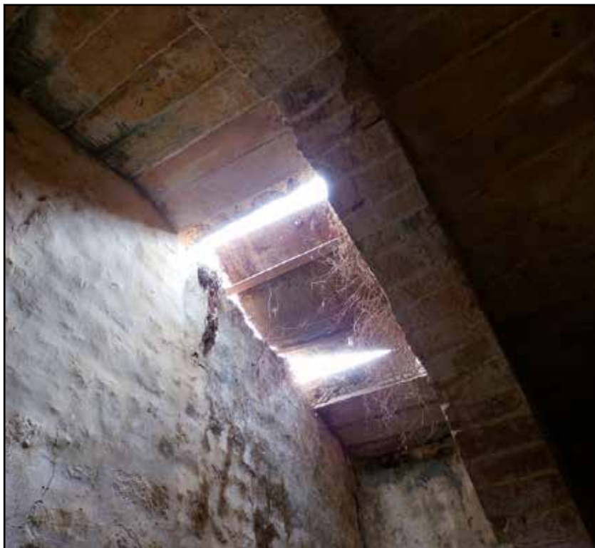
Part of the ceiling which has collapsed
