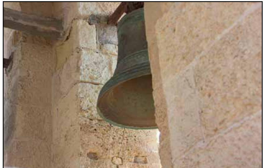
Damaged stone slabs precariously support one of the bells
