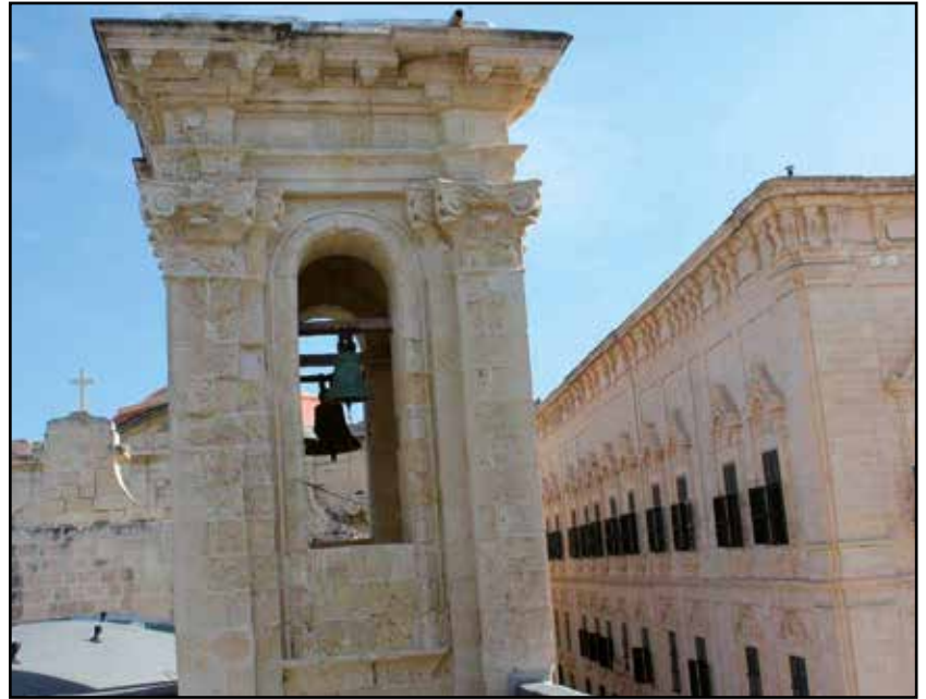
Prior to restoration - the carved belfry showing deteriorated masonry
